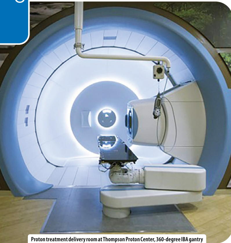
Proton treatment delivery room at Thompson Proton Center, 360-degree IBA gantry
